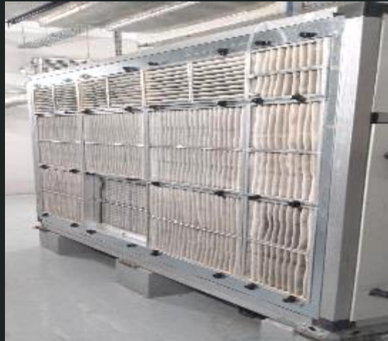
MERV Filters in AHUs
